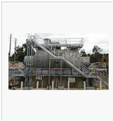
Side view of the condenser unit
