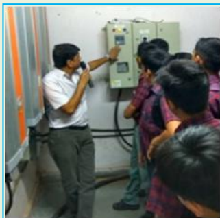
(Solar Control Panel)
